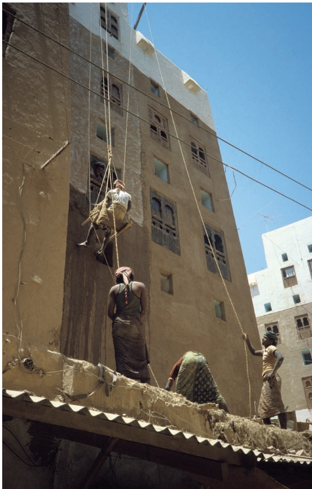
FIGURE 7.16 Plastering Work of the Façade of the Tower Houses. CREDITS: CHRISTIAN DARLES.
